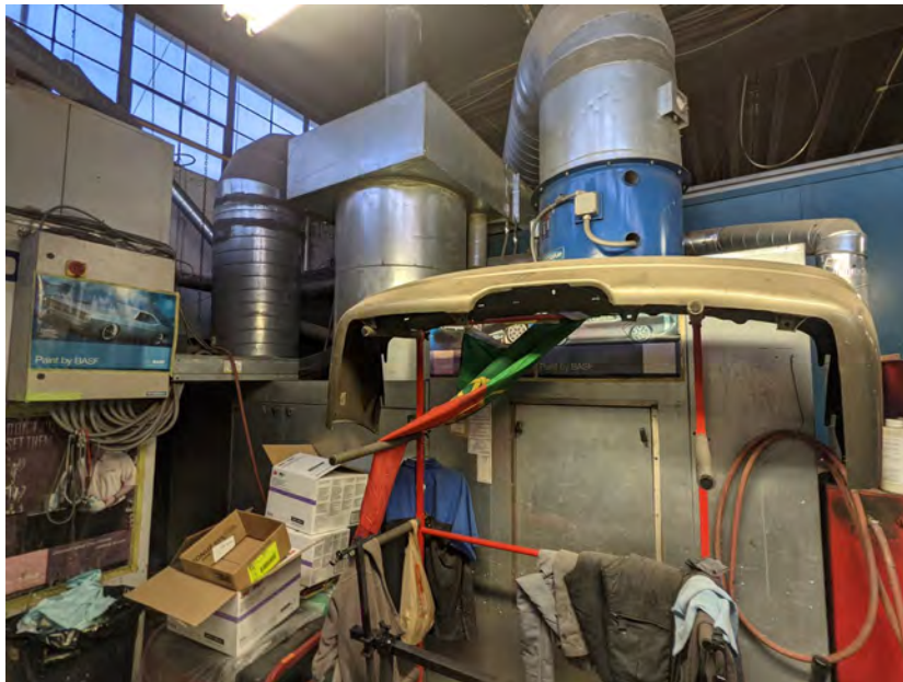
Photo 28 – Exhaust for the paint booth
