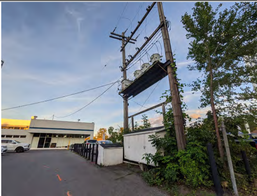
Photo 11 - Suspended transformers, westside parking lot entrance, adjacent to New Orchard Ave, facing northeast
