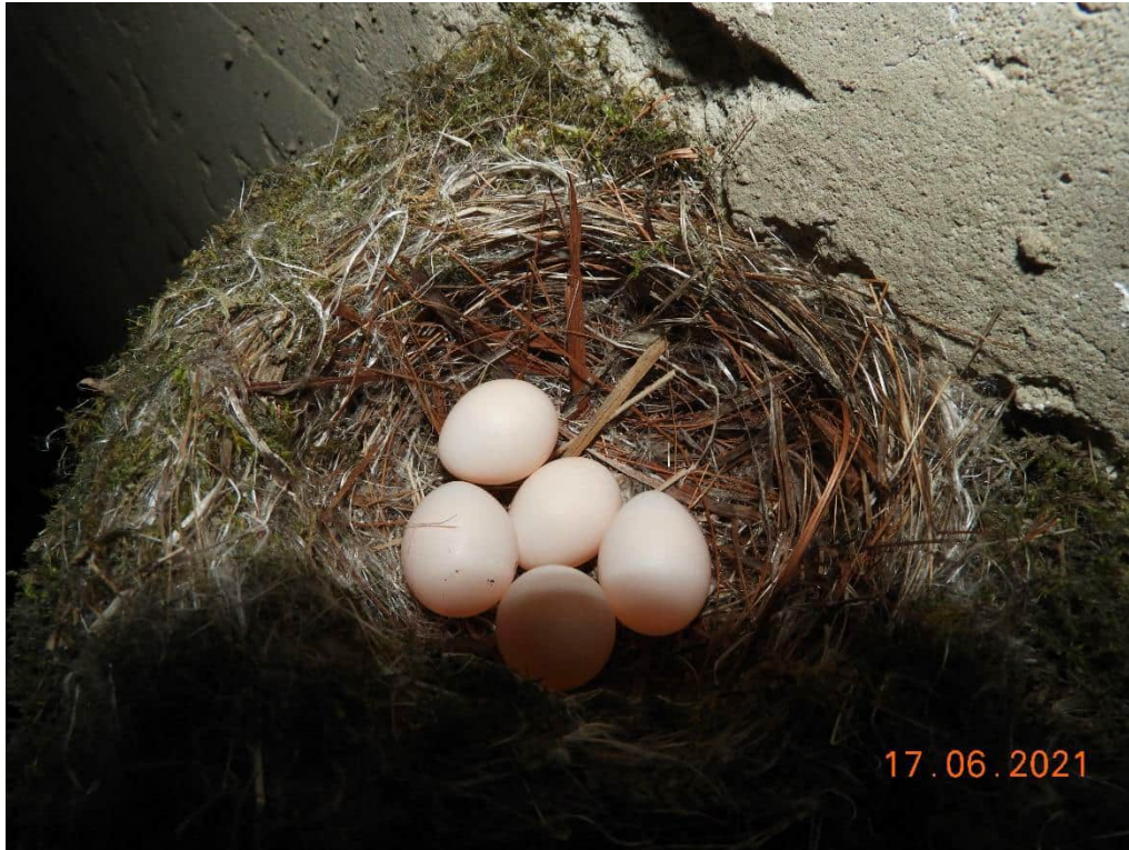
Photo 19: An active Eastern Phoebe ( Phoebe sayornis ) nest with eggs observed within the decommissioned railway culvert directly adjacent to the eastern extent of the study area. 17 June 2021.
