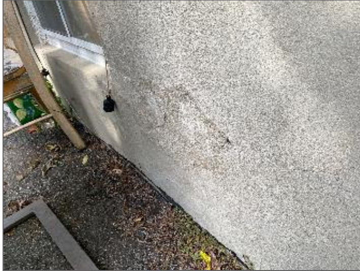
Photo 9 – Patching, inferred to be for a former heating oil AST, observed along the exterior elevation of Site Building B.
