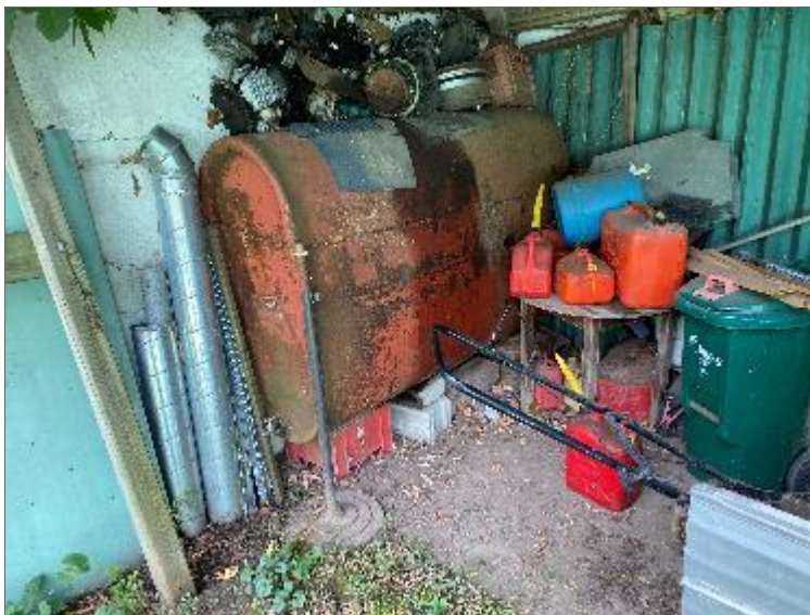
Photo 10 – AST observed beneath a covered storage area adjacent to the garage west of Site Building B.
