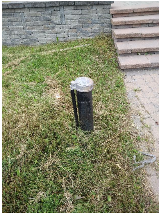
Photo 9: On-site well, front of office building.
