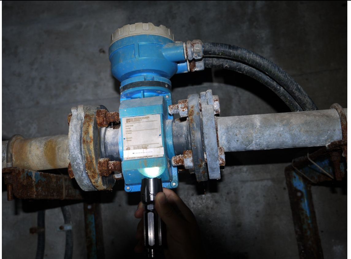
Photo 1: Flow meter: Endress + Hauser ProMag F
