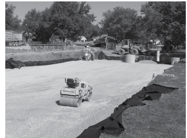
Place clean, crushed, angular stone foundation 6” (150 mm) min. Compact to achieve a flat surface.
