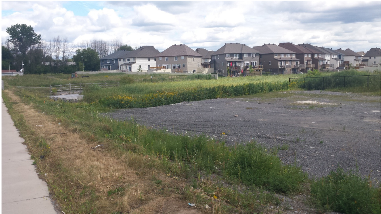
Photograph 7: View of 110, 88, and 80 Cope Drive, looking northeast. Mahoney Creek is present at the centre of the photo, and construction equipment is just visible on 80 Cope Drive, at centre left.
