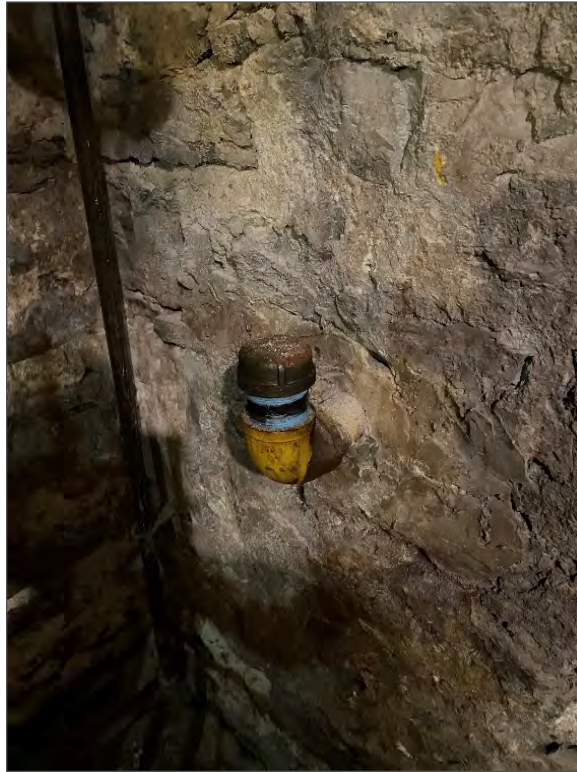
Photo 9 – Pipe indicating the presence of a former AST located in the basement of the Site Building.
