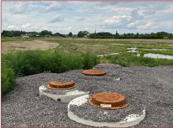
Photograph 9: Four OGS units observed on the northernmost portion of the Site and South of the stormwater discharge pond.
