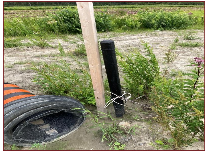
Photograph 6: One of multiple utility access points for future services across the Site.
