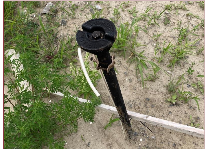
Photograph 8: One of several groundwater shutoff valves observed across the Site.
