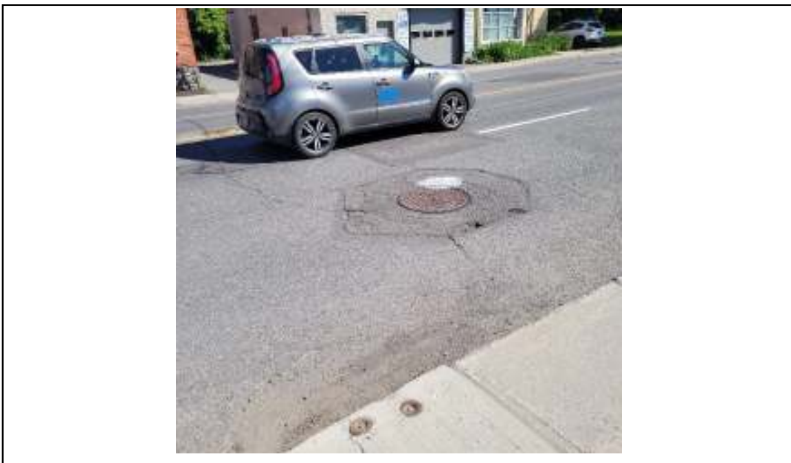
Photograph 26: Storm water manhole on Hawthorne Avenue, water service valves in sidewalk in front of 20 Hawthorne with former automotive service center across street at 25 Hawthorne.
