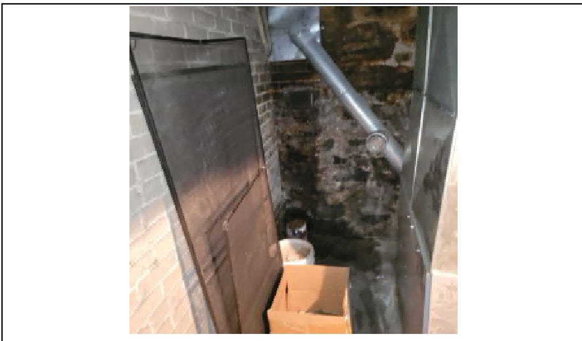
Photograph 14: Natural gas furnace and south-east basement wall of 16 Hawthorne. Staining on wall and floor appears to be water.
