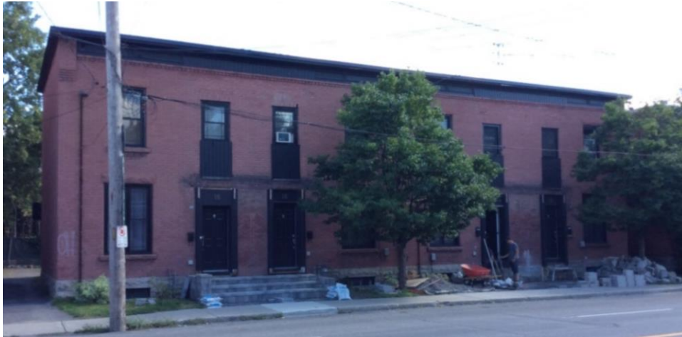
Figure 4: Street view of 12 Hawthorne the subject of this report. The property consists of four townhouses set on 6.m wide lots. The photo dates from circa 2016-2020. The entrance steps are being rebuilt and the existing entrance awnings have yet to be installed. Source: City of Ottawa
