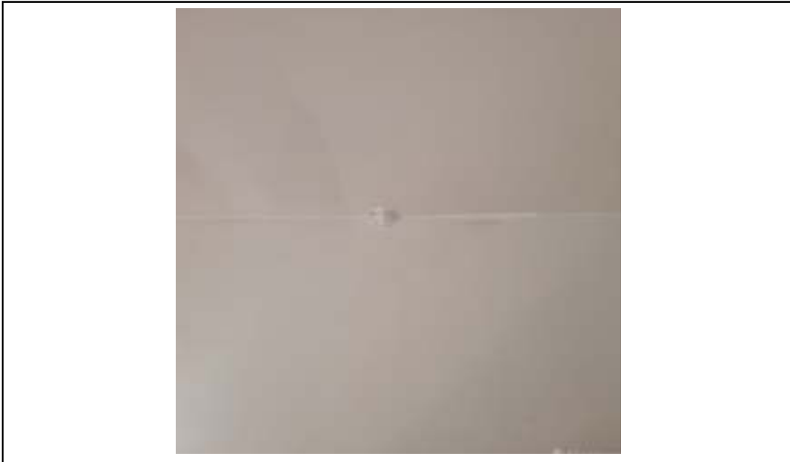
Photograph 9: West wall and ceiling of kitchen in 14 Hawthorne, note main sewer drain in corner of wall/ceiling.
