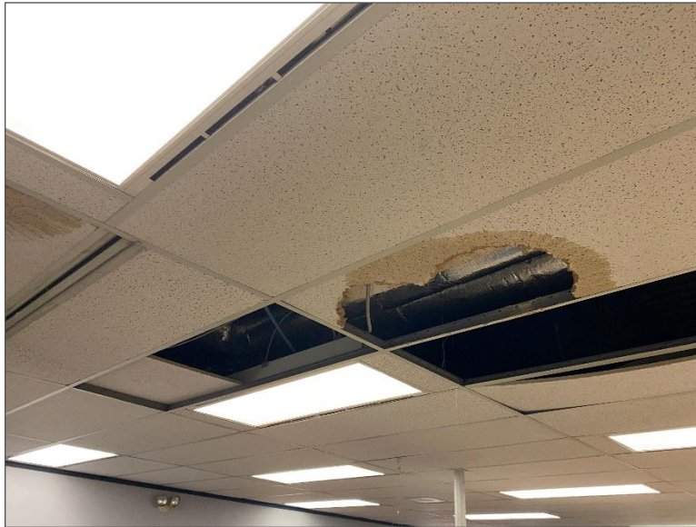
Photo 9 – Stained ceiling tiles located within the office portion of the Site Building.
