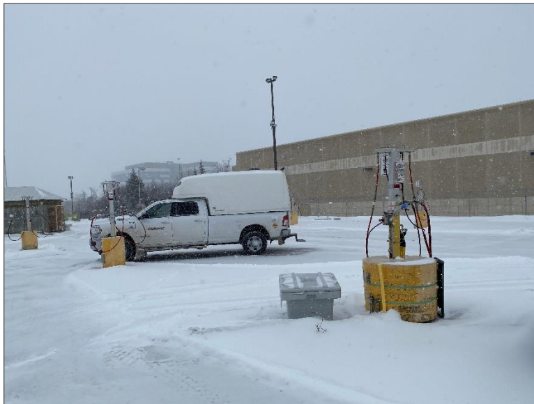
Photo 14 – Natural gas fuel pumps.
