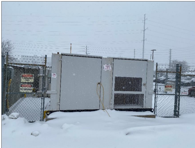
Photo 10 – Natural gas fuelling station.
