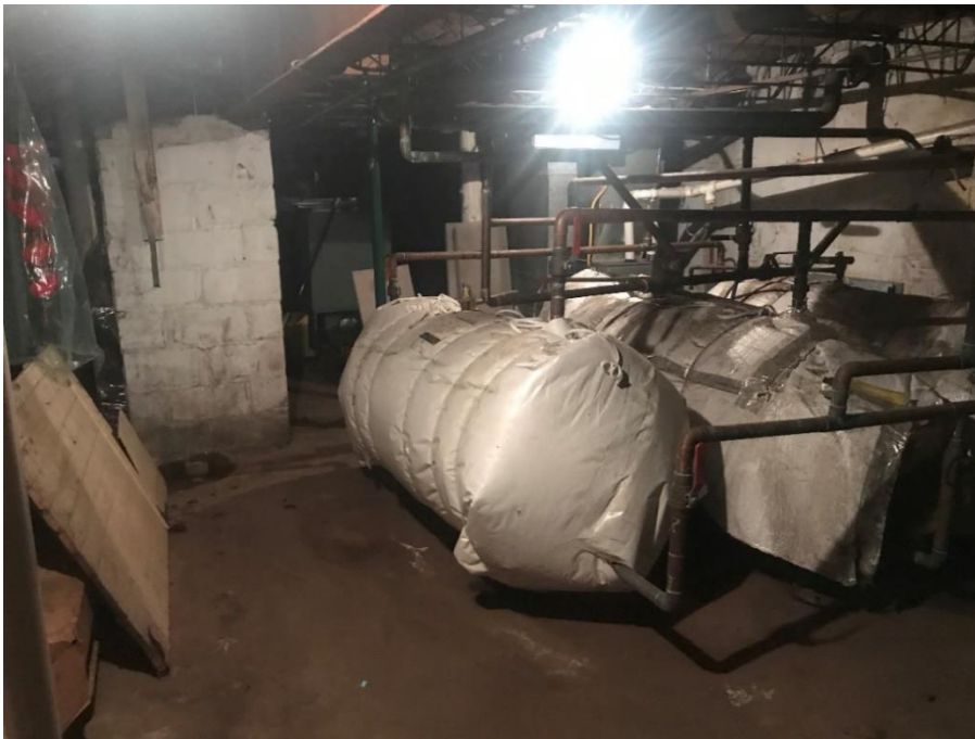
Photograph 24: Site building basement, hot water tanks (April 6, 2021).
