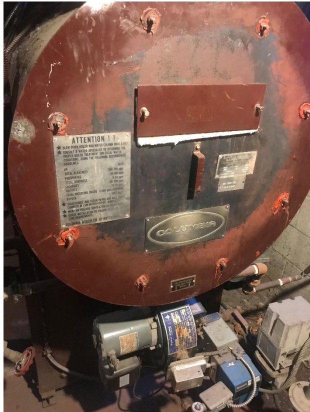
Photograph 28: Boiler in basement of Site building (April 6, 2021).
