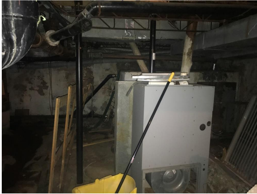
Photograph 25: Heating system in basement of Site building (April 6, 2021).
