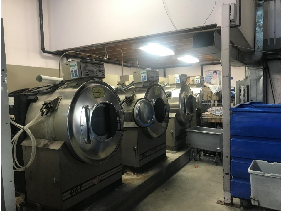
Photograph 15: Site building interior, commercial laundry machines (April 6, 2021).
