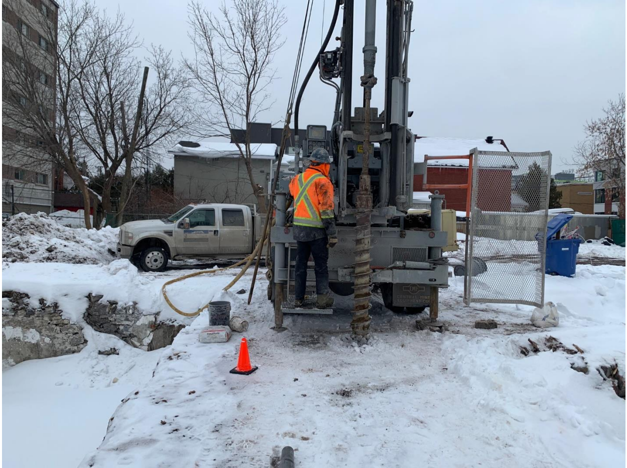
Image 2 – Monitoring Well 1, facing east (later decommissioned)
