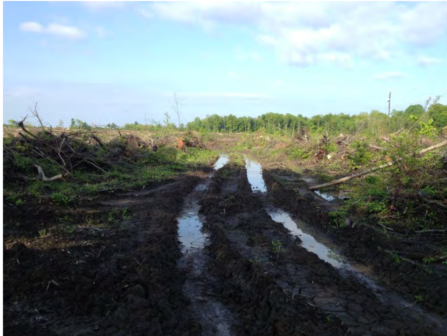
Figure 60: Evidence of machine damage during grubbing in Operation 11 (D368).
