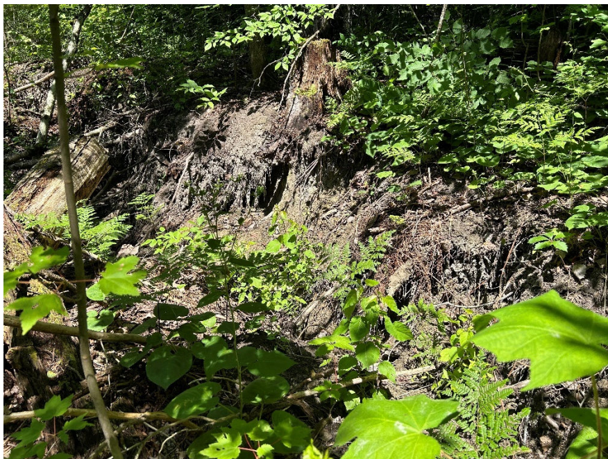
Photograph taken at the downstream extent of R3 facing the top of a large slump. The slump was located on the right bank and carried debris over the channel.
