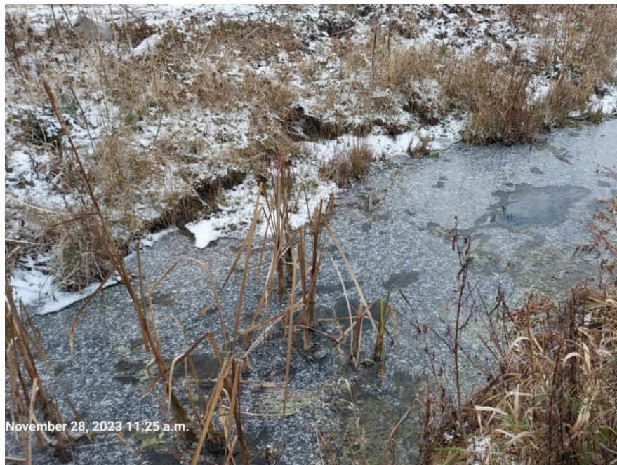
Photograph taken facing the left bank at the downstream extent of R1 . Minor scour was observed along both banks.
