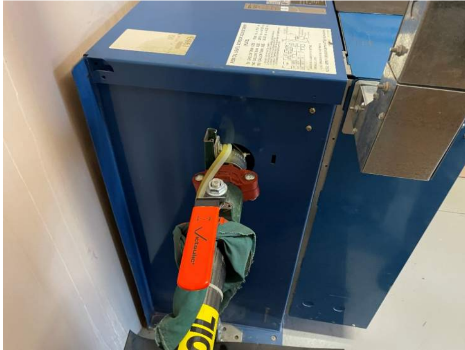
Photo 7: Hydraulic oil storage tank and pump for elevator system in 603 March Road.
