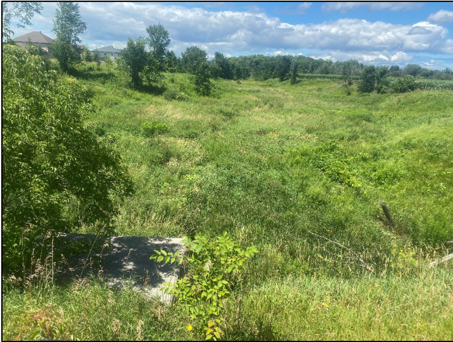
1. Wilson Cowan Drain - Facing downstream, Wilson-Cowan Drain and valley from Bankfield Road
