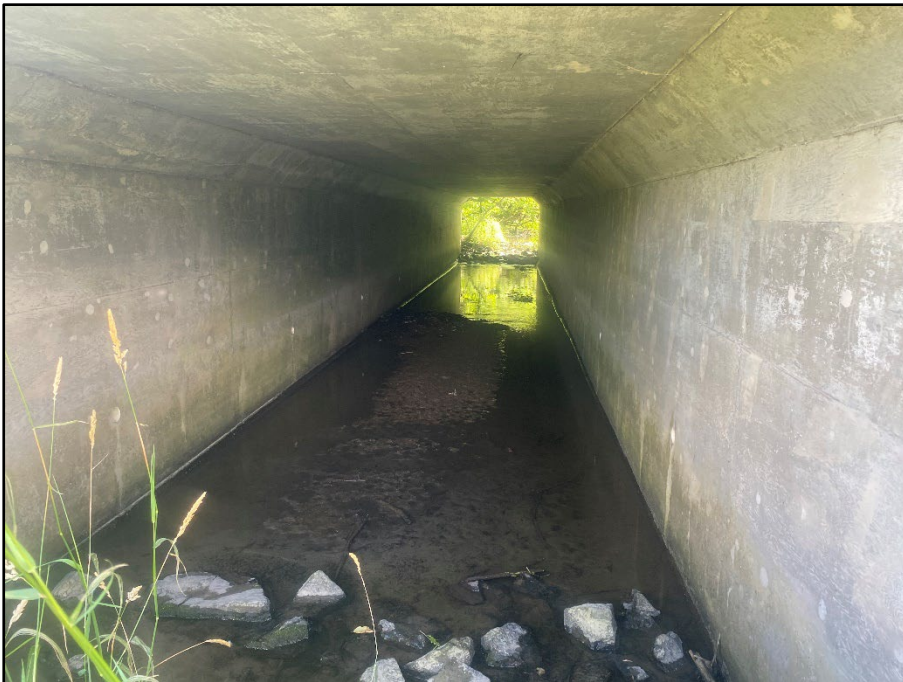
2. Wilson Cowan Drain - Facing upstream from outlet of culvert passing under Bankfield Road
