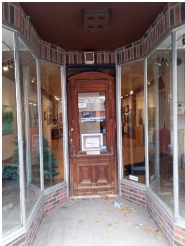
Figure 18: Although the shopfronts have been dramatically altered elements such as the recessed shopfront at 227 Bank Street are still evident. The leaded transom and vaulted arch have been covered over. Based on the 1950 photo it would appear that the three shopfronts at 215, 217 and 219 were similar with recessed entrances and decorative transoms.
