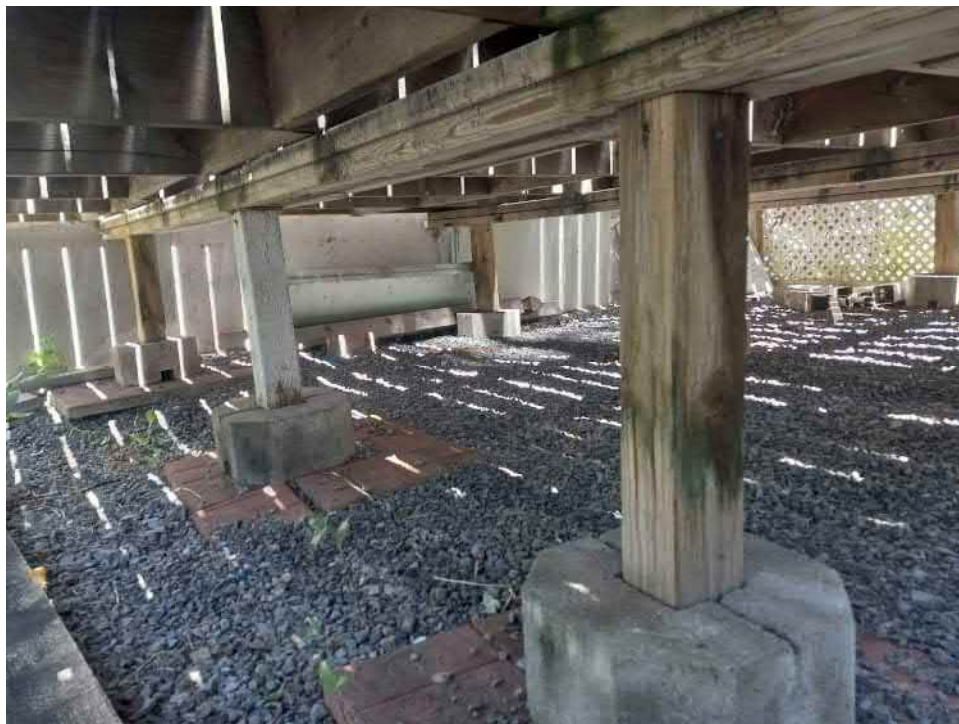
Photo 8: View of materials underneath backyard deck.
