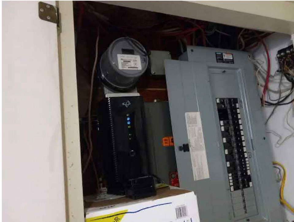
Photo 13: Electrical panel within one residential unit.
