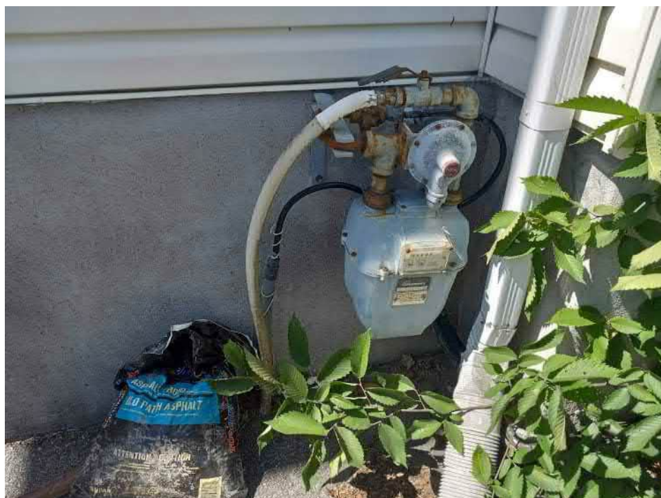
Photo 10: Natural gas hookup located along eastern side of the building.
