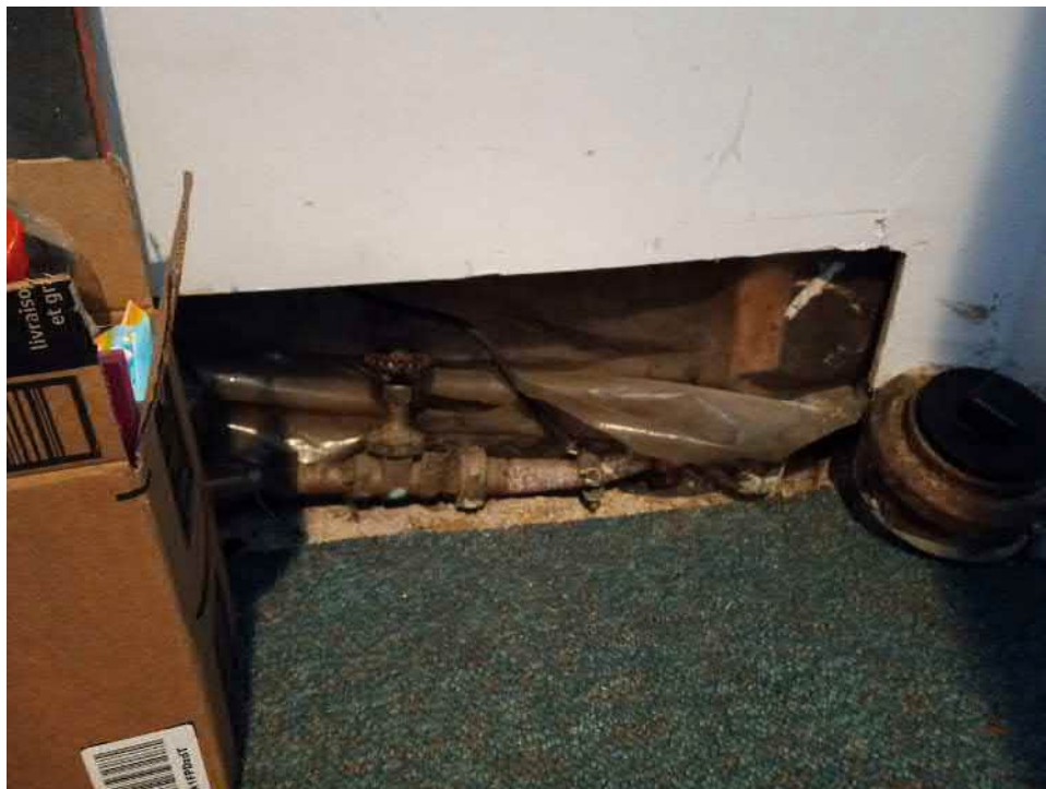
Photo 11: Water pipes located in basement level of one residential unit.
