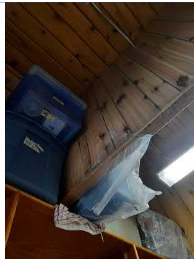
Picture 4 – Patched portion of ceiling in site building that has been reported by staff to have leaks in the past
