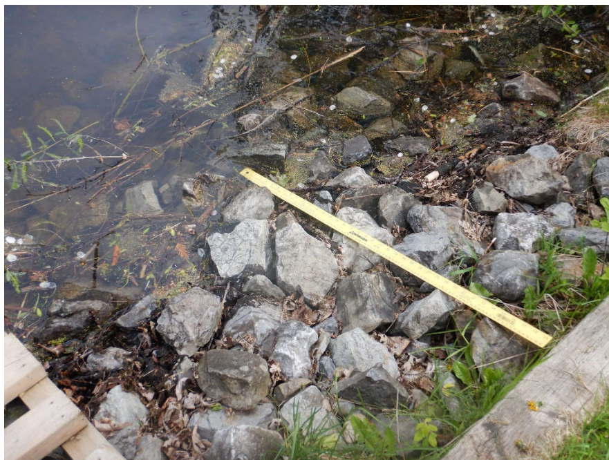
Photograph taken at the downstream extent of the subject lands. The remainder of the bank was composed of 10-20 cm rip rap.
