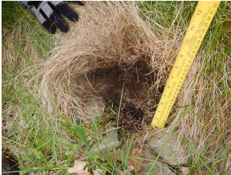
Erosion blanket observed at several locations along the bank under the rip rap.
