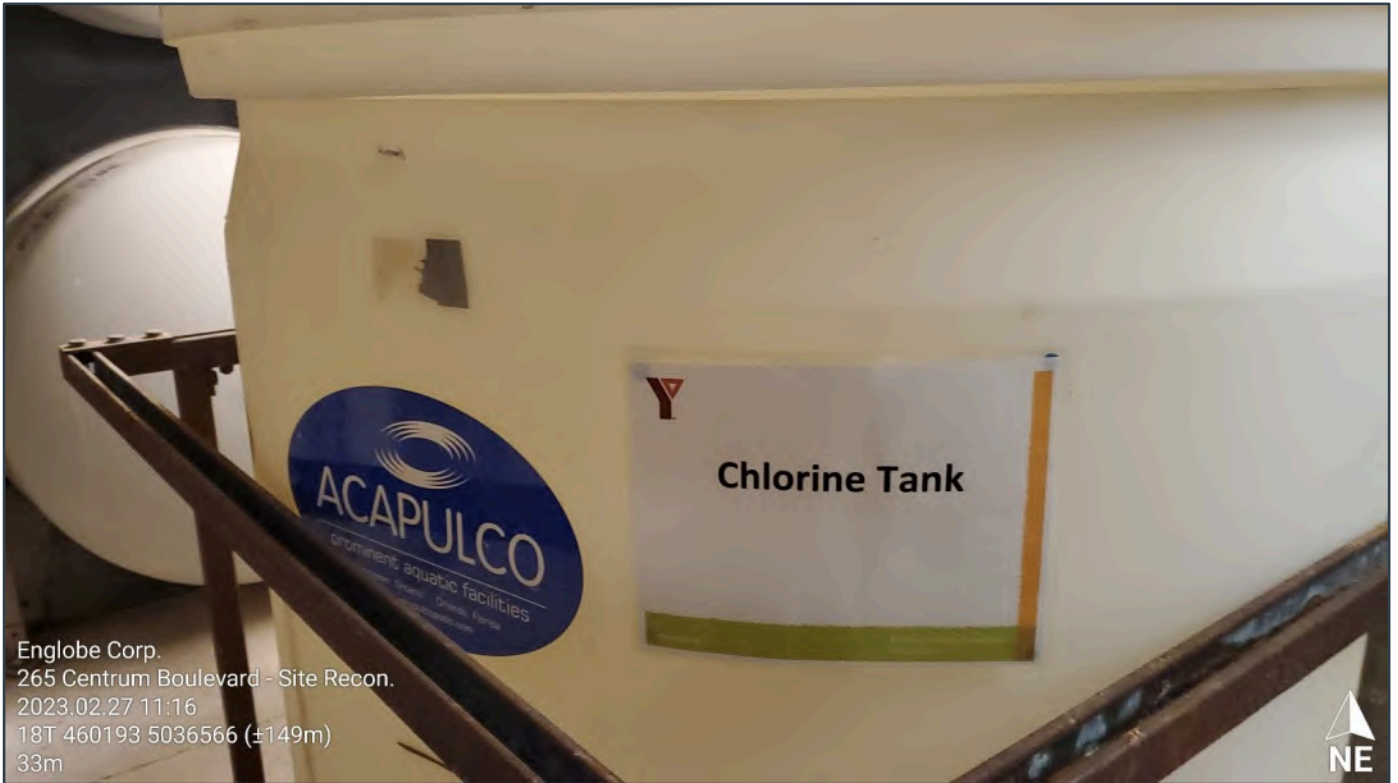
Site Photograph 7: Overview of the plastic chlorine tank (empty) in the pool valve room (basement).
