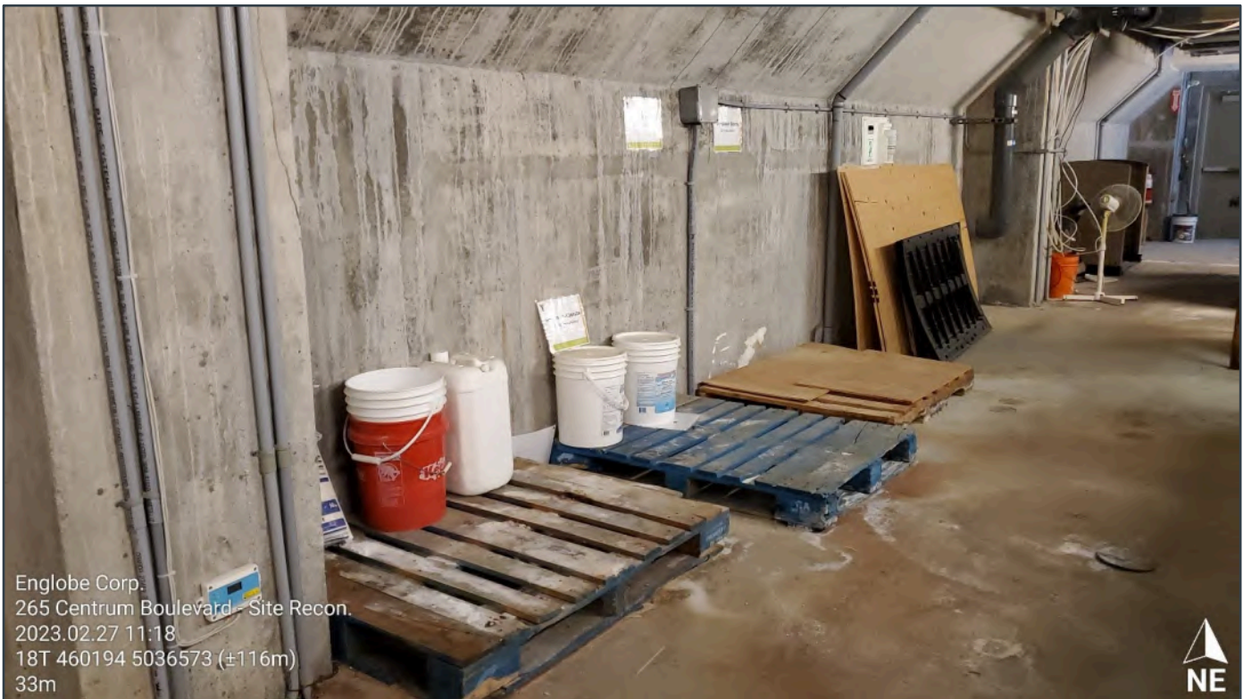
Site Photograph 6: Overview of the pool chemical storage area in the pool valve room (basement).
