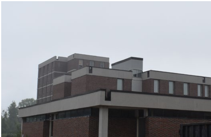
Figure 24. Added volume at upper levels of Building J, viewed from southwest of Building I (ERA, 2021).
