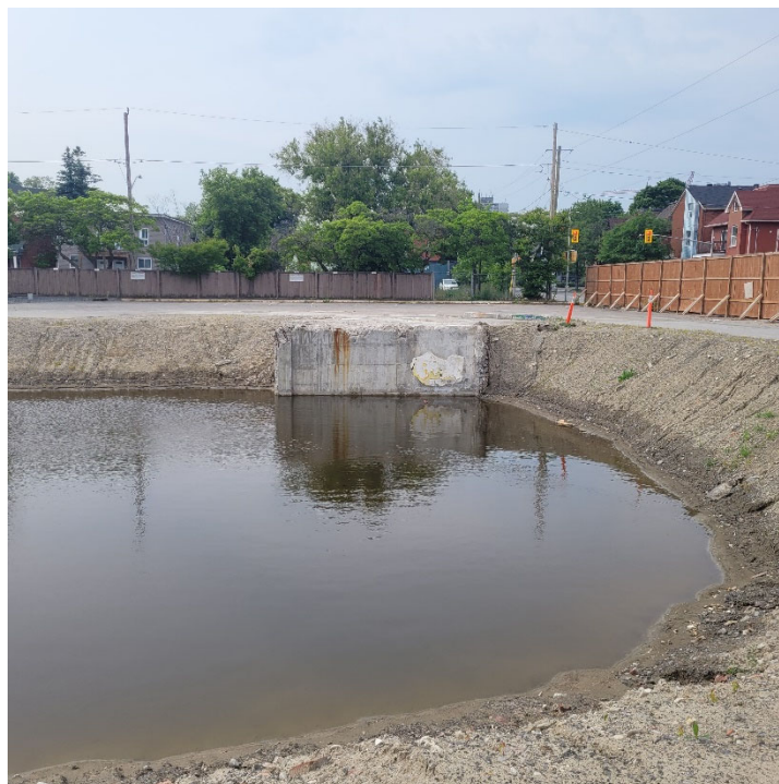
Photograph 2: View of excavation of the former building footprint which had filled with water. The foundation wall adjacent to the diesel UST was left in place. View is looking north.
