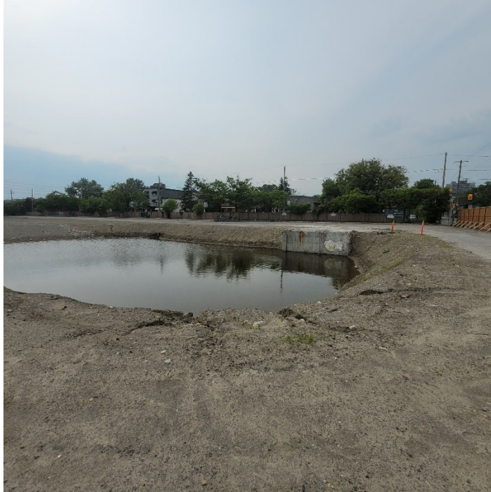
Photograph 1: View of excavation of the former building footprint which had filled with water. The foundation wall adjacent to the diesel UST was left in place. View is looking northwest.
