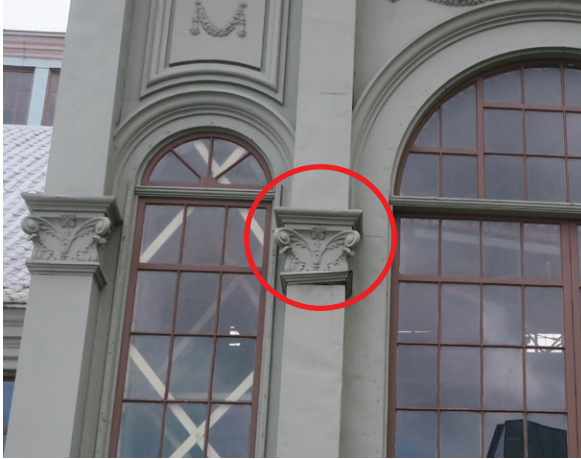
North entrance pavilion: damaged sheet metal capital details from ice and snow impacts (ERA 2023)
