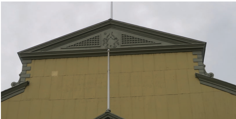
Dented metal panels edges and patches of repair above the east entrance pavilion (ERA 2023)
