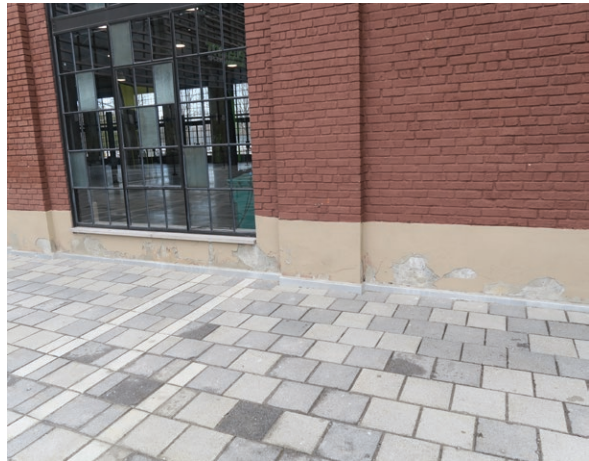
Delaminated material and paint flaking base on west elevation of exhibition hall (ERA 2023)
