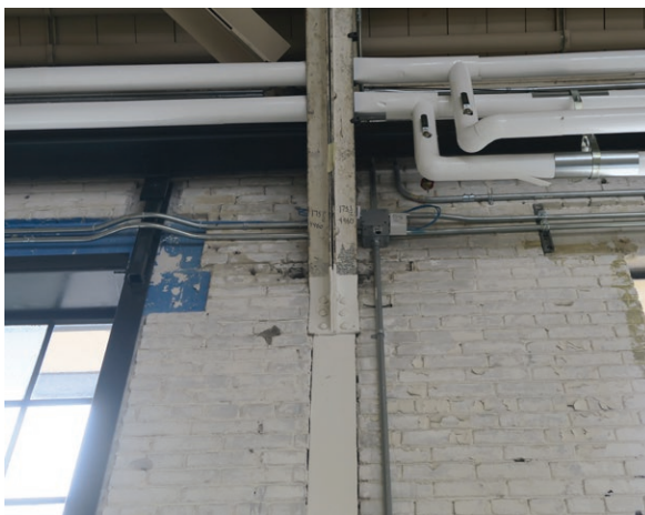
Deteriorating brick walls on the west wall of the exhibition hall at the truss (ERA 2023)
