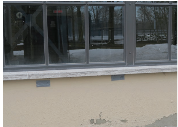
Dry glazing putty on bottom window panes (ERA 2023)
