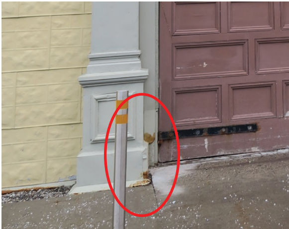
North entrance pavilion: rusted base and dented metal on pilaster adjacent to doors (ERA 2023)
