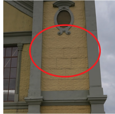
Rust present at perimeter of metal panels on northeast corner turret (ERA 2023)
