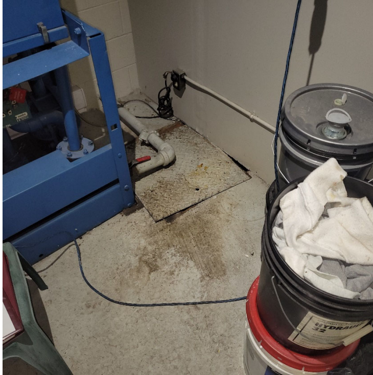
Photograph 7: View of the hydraulic reservoir (blue), floor sump pit and pails of stored hydraulic oil in the elevator room.
