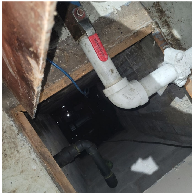
Photograph 8: View of the floor sump pit adjacent to the elevator reservoir in the elevator room.
