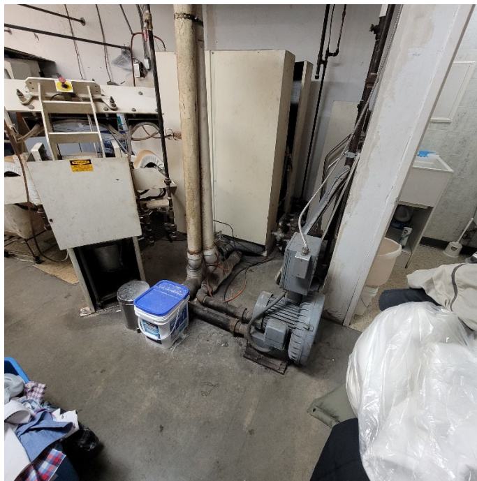
Photograph 6: View of the dry cleaning equipment on the interior of the dry cleaner unit. View is looking west.
