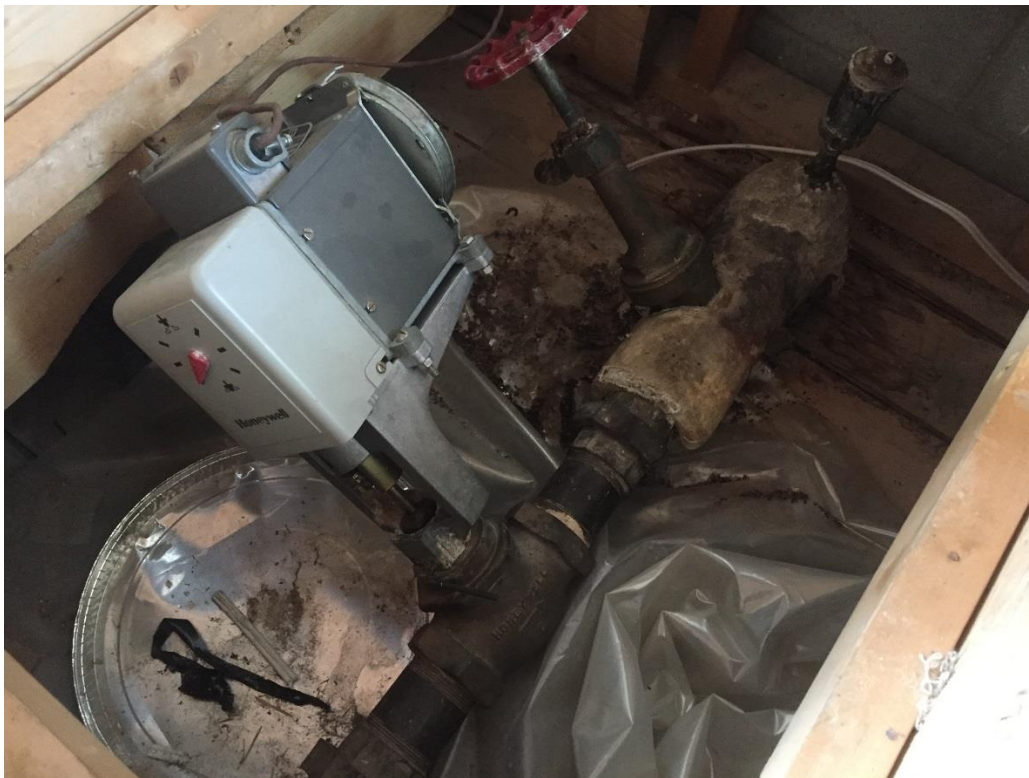
Photograph 2: Pipe lagging in poor condition. Located in the church balcony floor panel.
