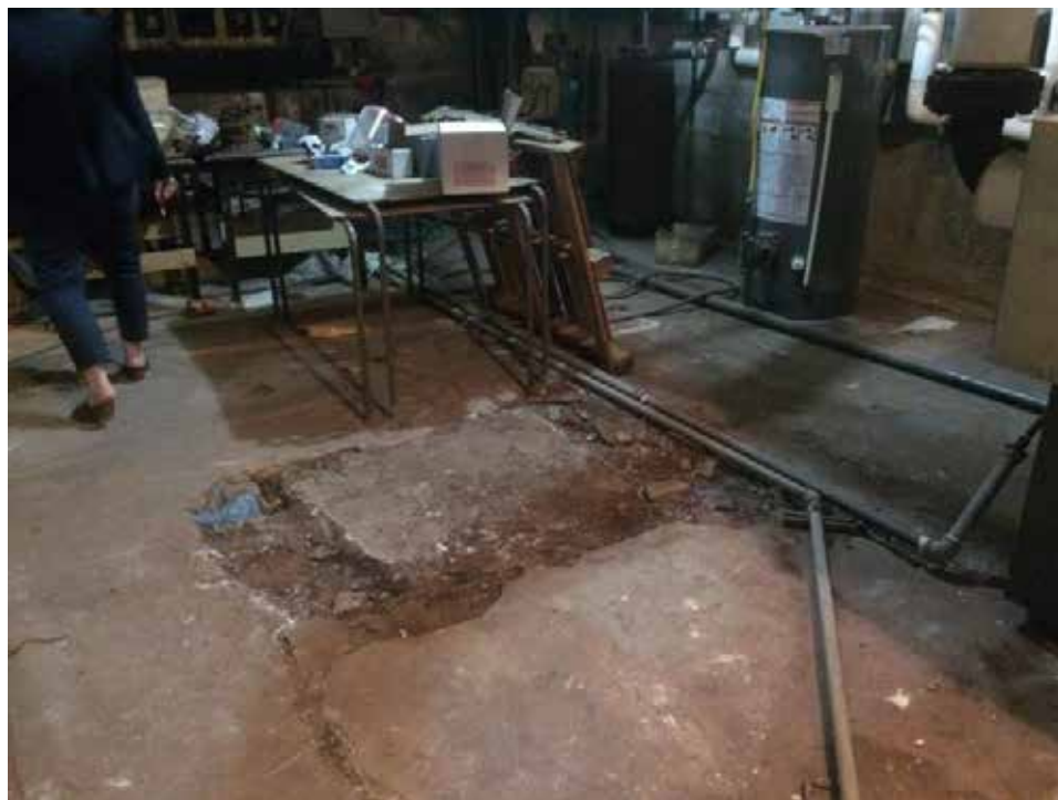
Photograph 13. View of the mechanical room, located in the basement of the church
