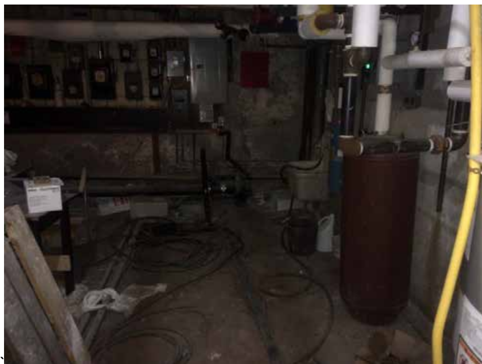
Photograph 12. View of the mechanical room, located in the basement of the church
