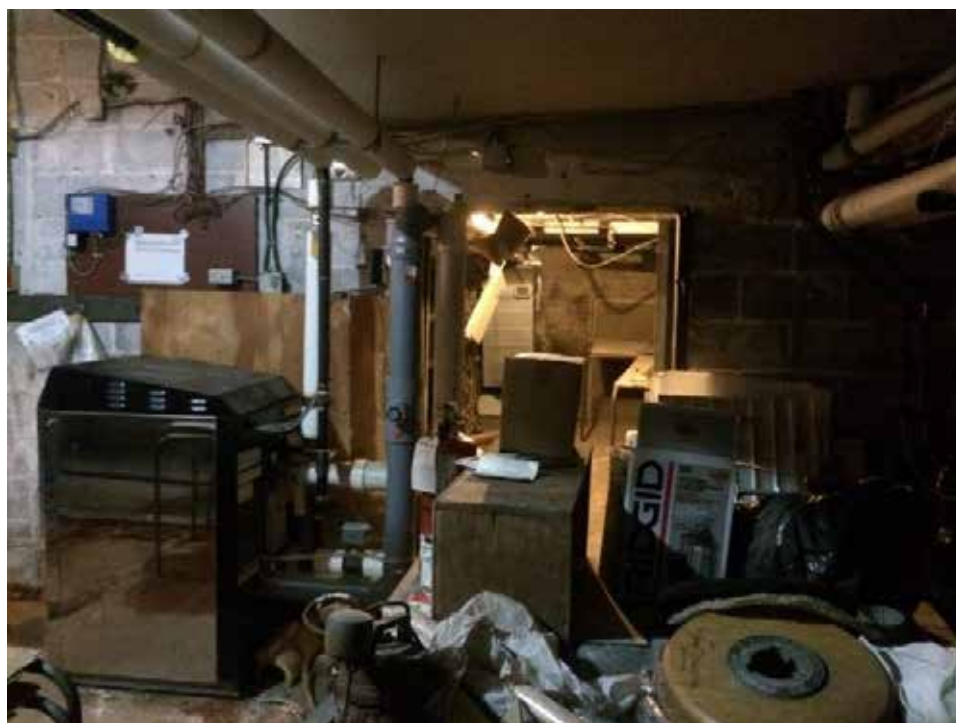
Photograph 14. View of a furnace, located in the mechanical room of the church
