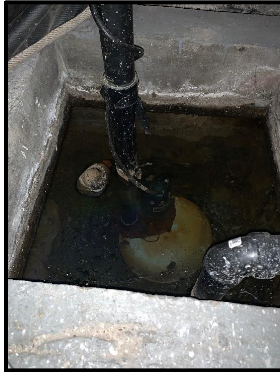
Photograph 5: View of the sump pit with sheen located in the basement of the 1137 Ogilvie Road.
