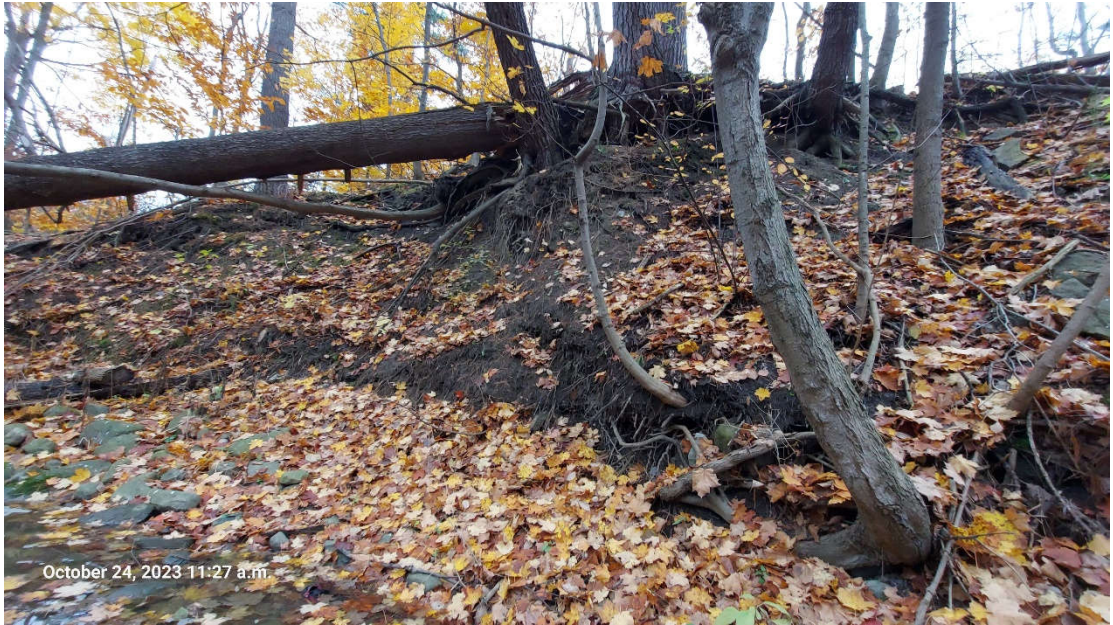
Photograph taken facing southwest at the right bank. A large cutface in the valley wall (approximately 5-7 m tall, 10-15 m long) was observed. Young J-hooked trees and exposed roots were present.
