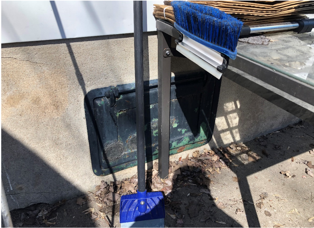
Photograph 3: View of the former coal chute from the exterior of the dwelling, looking north.
