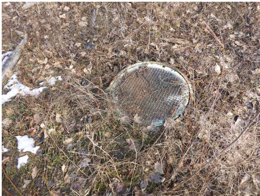
Image 6: Manhole located in the northwest corner of the study area, view north.
