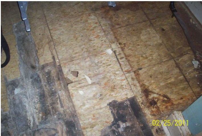
Photo No. 1 – Asbestos Containing Vinyl Floor Tile, Sample Group 72-AS-022511-01
