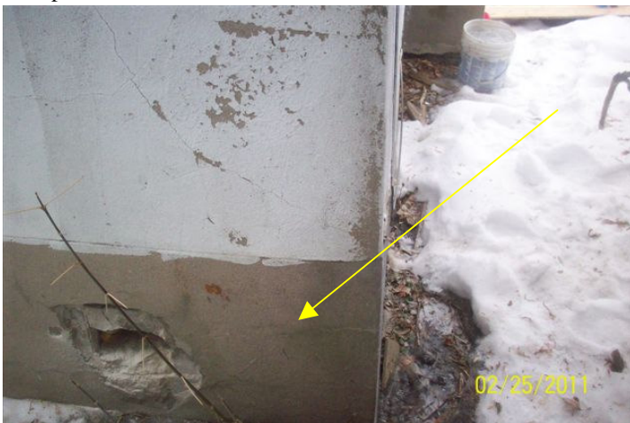
Photo No. 5 – Exterior Parging located on foundation and rear exterior wall, Sample Group 72-AS-022511-05
