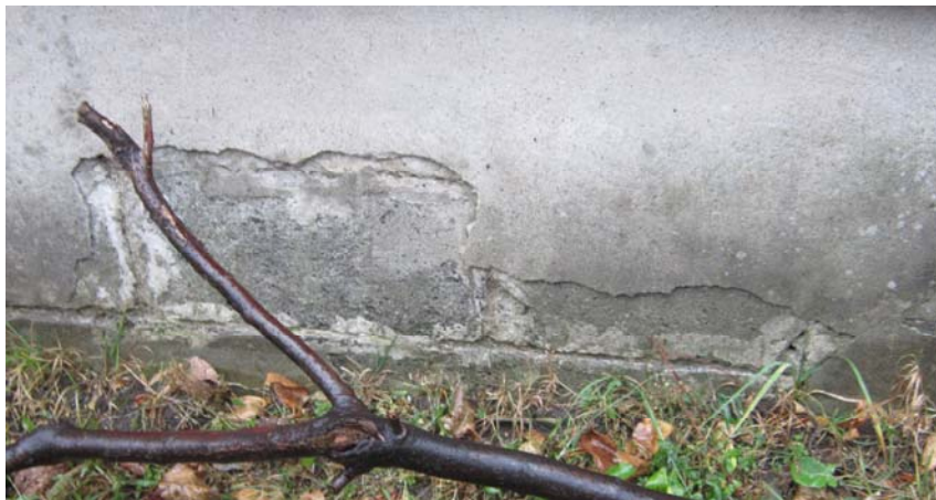
Photo 1 - Cracked Parging & Concrete Block
