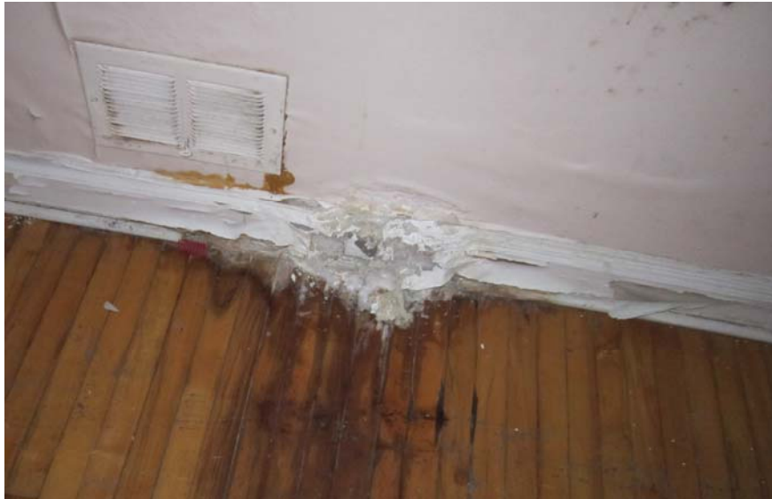
Photo 4 – Interior Water Damage
