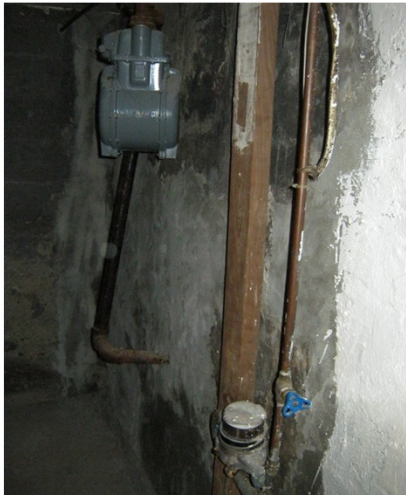
Photo: F01085_B202001 Domestic Water Distribution_Sept 2011_1 Description: Incoming water main and metre at Unit 153-2.
