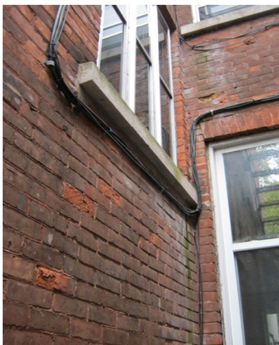
Photo: F01085_B201001 Exterior Closure - Brick_Sept 2011_1 Description: Spalled brick masonry.
