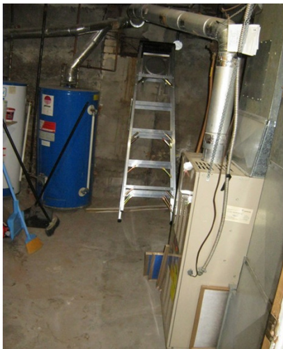
Photo: F01085_D302003 Furnaces_Sept 2011_1
