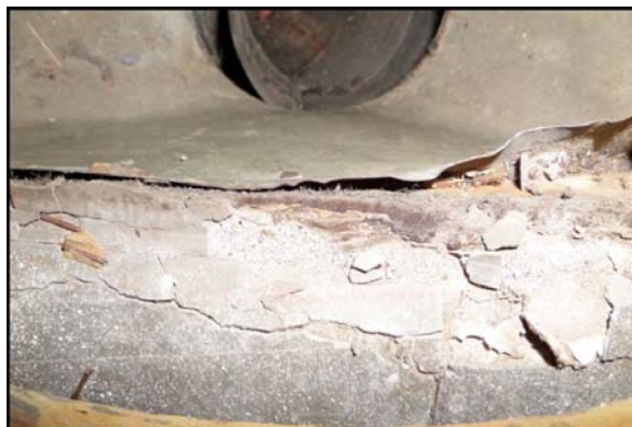
Photograph 3 – ASBESTOS CONTAINING flooring (dark brown) located at 1-151 Arlington Avenue, under the carpet in the 1 st Floor, North Bedroom.
