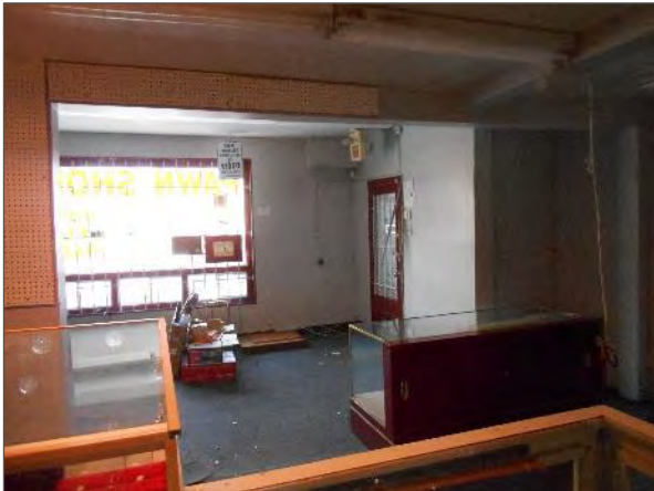
View of illuminated exit sign and emergency lights in the commercial unit on the northeast portion of the Site Building.
