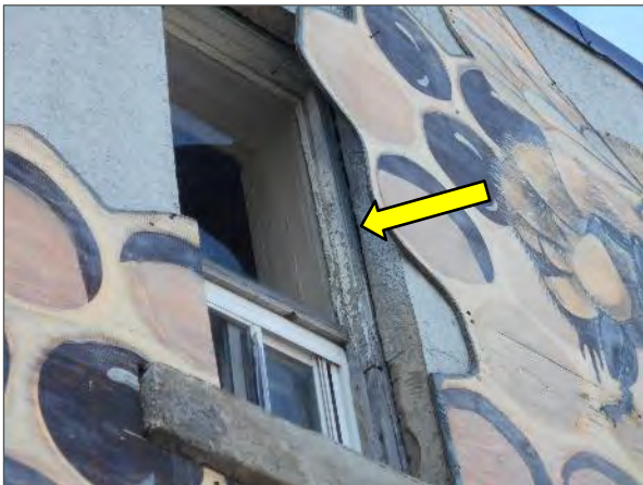
View of deteriorated window frame and sealant at perimeter of the window frame.
