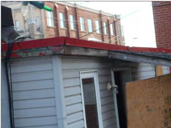
View of fascia wood rot on the two storey portion of the Site Building.
