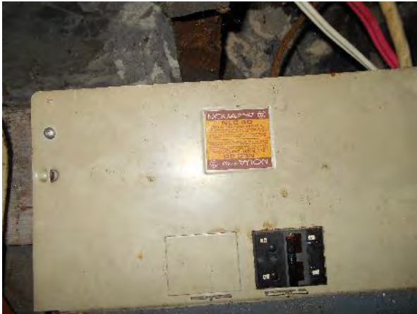
View of the electrical main disconnect switch in the basement.
