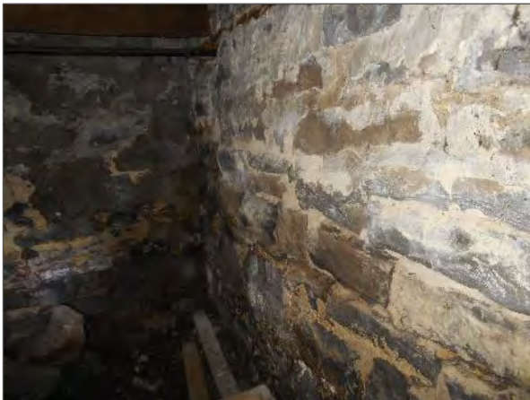
View of stone foundation wall within the basement area of the east portion of the Site Building.
