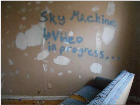
View of graffiti on the second floor apartment unit wall.
