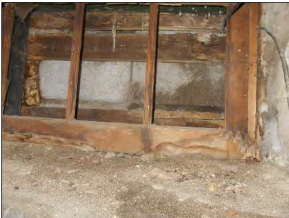
View of concrete block masonry foundation wall for the northwest portion of Site Building.
