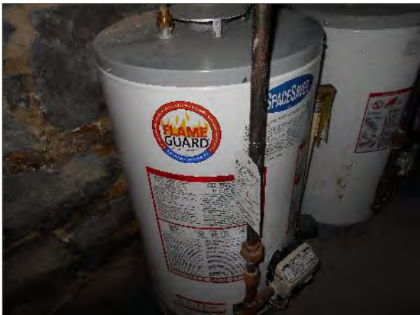
View of the hot water tanks within the basement of the Site Building.
