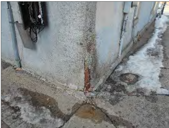
View of damaged and deteriorated stucco noted on the southeast corner of the Site Building.
