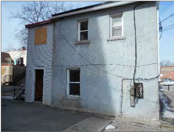
General view of the wall cladding on the south elevation of the Site Building.
