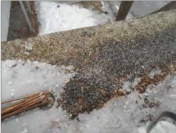
View of the BUR system atop the single storey portion of the Site Building.
