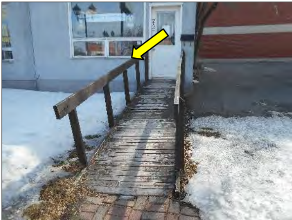
View of the wheel chair access ramp on the northwest corner of the Site Building.
