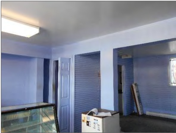
General view of the interior finishes within the commercial unit on the northwest elevation of the Site Building.
