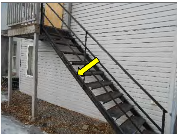
View of the metal stair case located on the west elevation of the Site Building.
