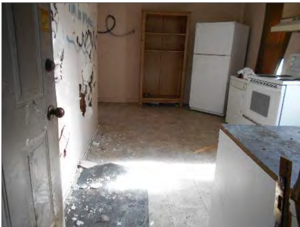
View of damaged drywall in the second floor apartment unit.
