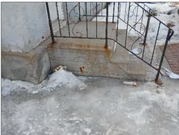
View of damaged pre-cast concrete steps located on the northeast corner of the Site Building.
