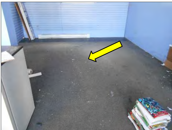
View of slab heaving in commercial unit on the northwest elevation of the Site Building.
