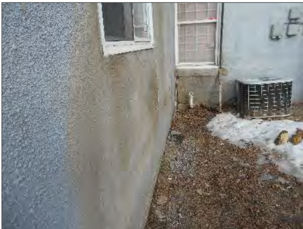
View of the stucco bowing noted on the west elevation wall.
