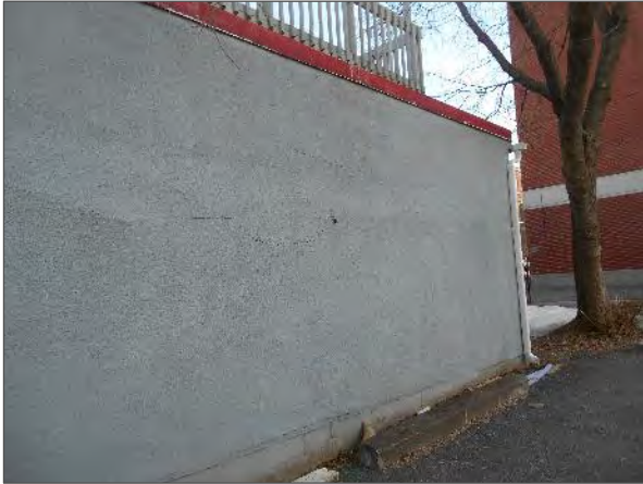
View of cracked delaminated stucco on the west elevation wall.
