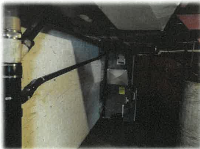
Photograph 9: View inside 20 Hawthorne at shared sewer line exiting 20 Hawthorne.
