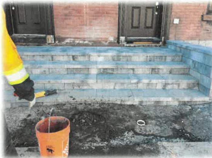
Photograph 6: View of front (north side) of 20 and 22 Hawthorne during the installation of MW13.
