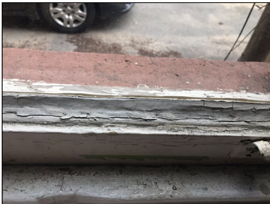
Photograph 11: main level, north wall window caulking
