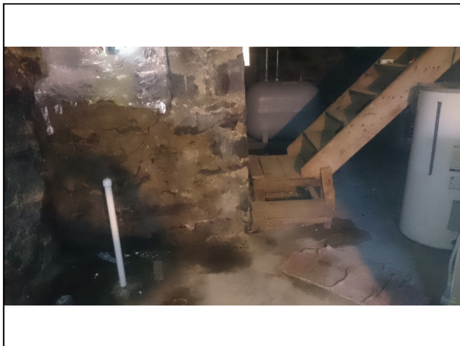
Photograph 8: Basement of 22 Hawthorne with current AST in basement and oil stain on foundation wall at left of picture from previous exterior AST leak.
