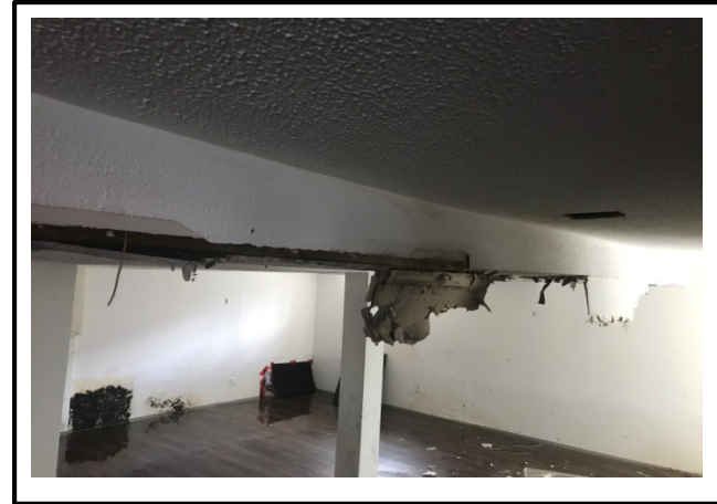
Photograph 2: Mould impacted drywall located in the basement.
