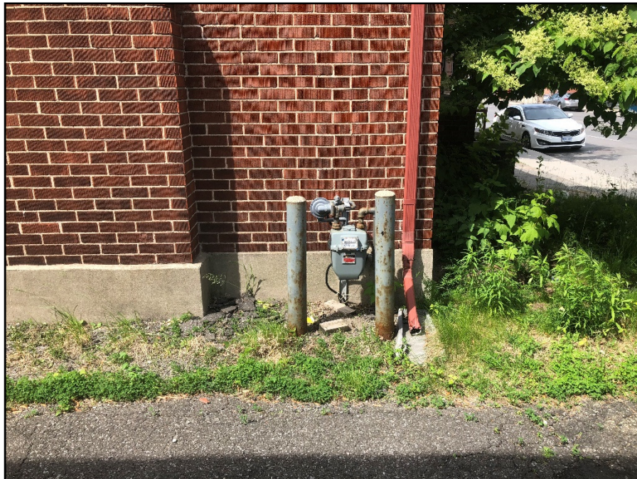
Photograph 3: Natural gas service on east wall, north end
