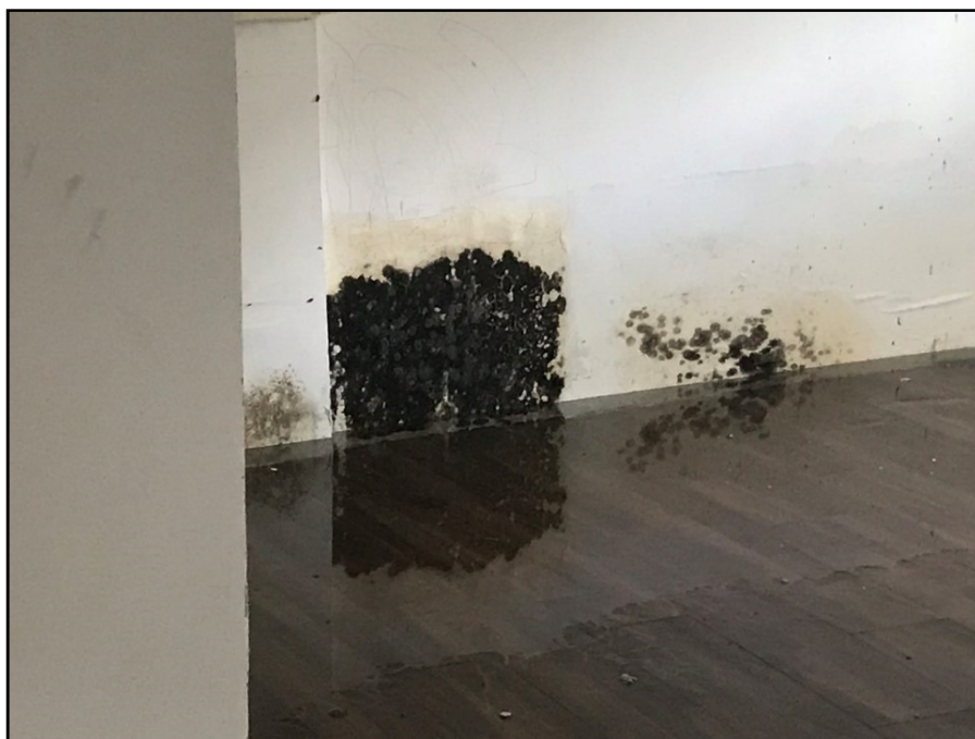
Photograph 16: Lower level of home with water present on floor and mould on drywall
