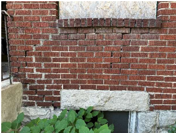
Photo 11: 281 Bell St - Exterior Brick damage – Step cracking
