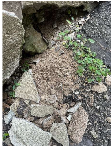
Photo 12: 273 Bell St - Concrete foundation deterioration at grade (exterior)
