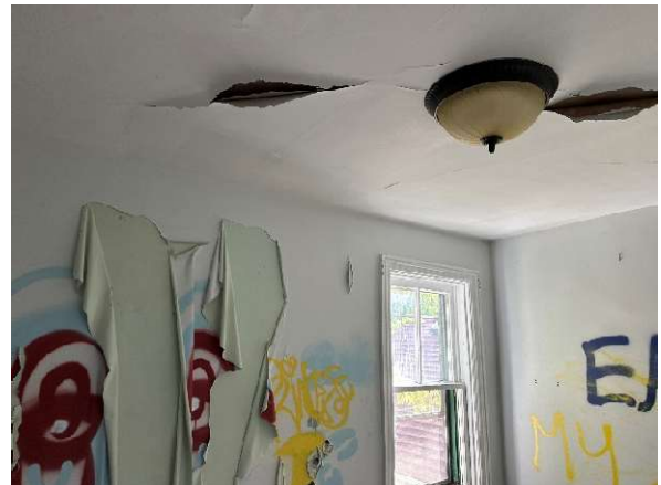
Photo 4: 281 Bell St - Interior paint peeling and ceiling damage
