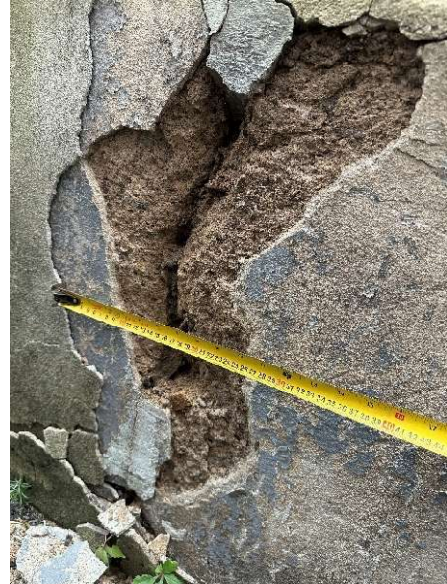
Photo 14: 273 Bell St - Concrete foundation large crack (exterior)
