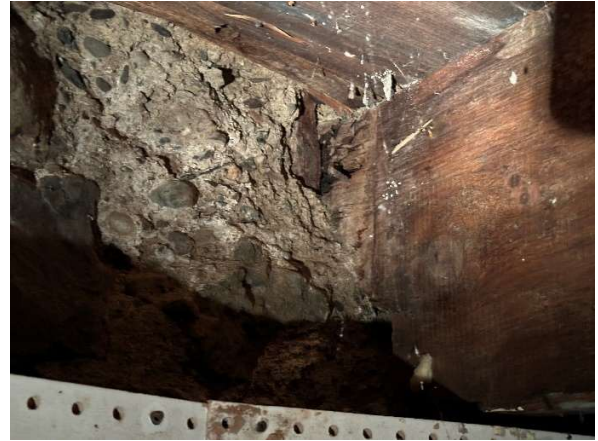
Photo 18: 275 Bell St - Wood beam Dry rot
