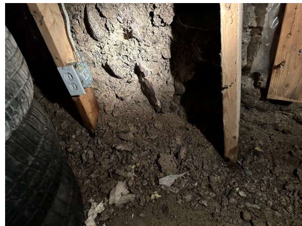
Photo 16: 275 Bell St - Concrete foundation deterioration (interior)
