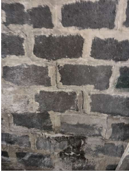
Photo 21: 277 Bell St - Step cracking in interior foundation wall
