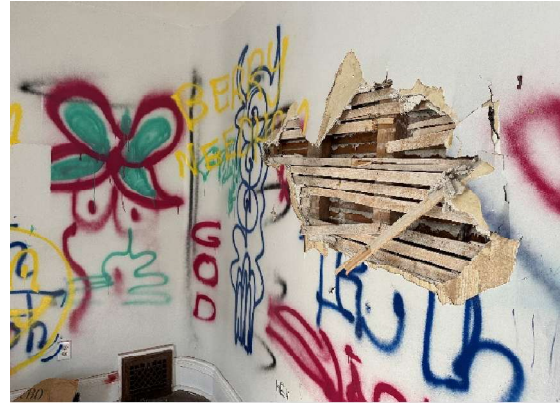
Photo 6: 281 Bell St - Interior wall damage
