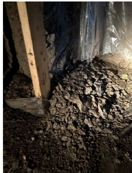
Photo 20: 275 Bell St - Foundation wall debris at base of wall (interior)
