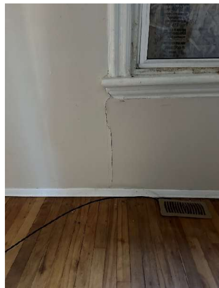
Photo 8: 275 Bell St - Interior cracking in finishes at window
