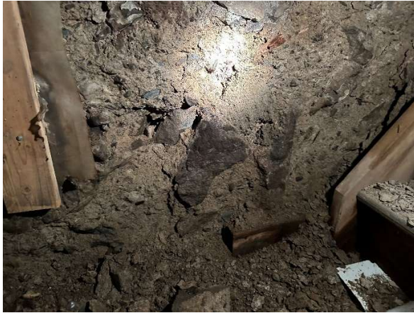
Photo 17: 275 Bell St - Concrete foundation deterioration (interior)
