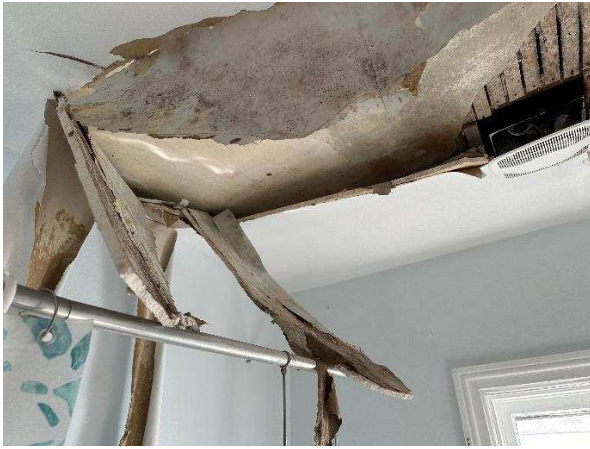
Phot 5: Interior Failed Ceiling
