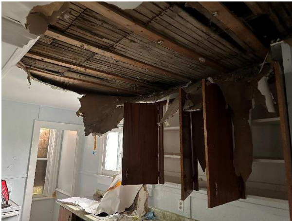
Photo 3: Failed Interior Ceiling
