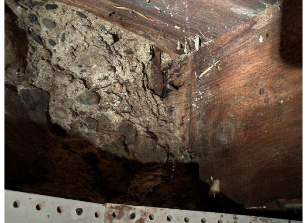
Photo 18: Wood beam Dry rot
