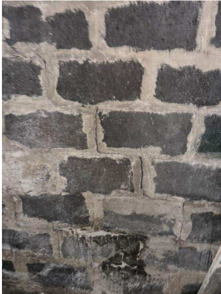
Photo 21: Step cracking in interior foundation wall
