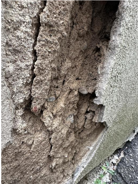
Photo 13: Concrete foundation deterioration (exterior)
