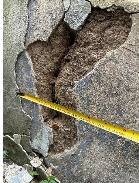
Photo 14: Concrete foundation large crack (exterior)
