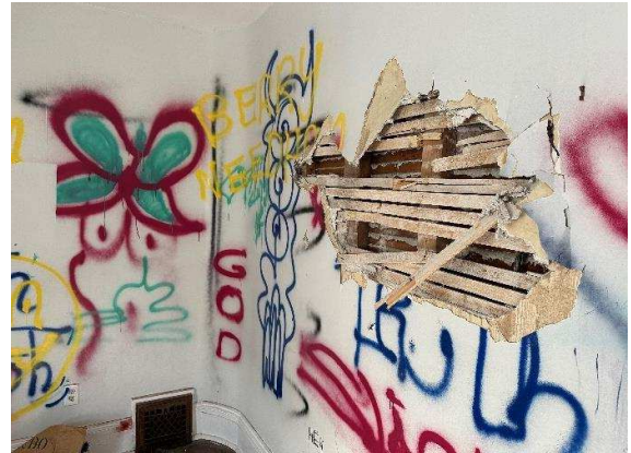
Photo 6: Interior wall damage
