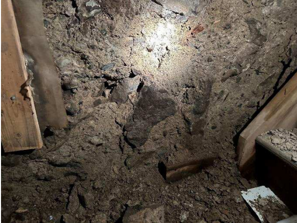
Photo 17: Concrete foundation deterioration (interior)
