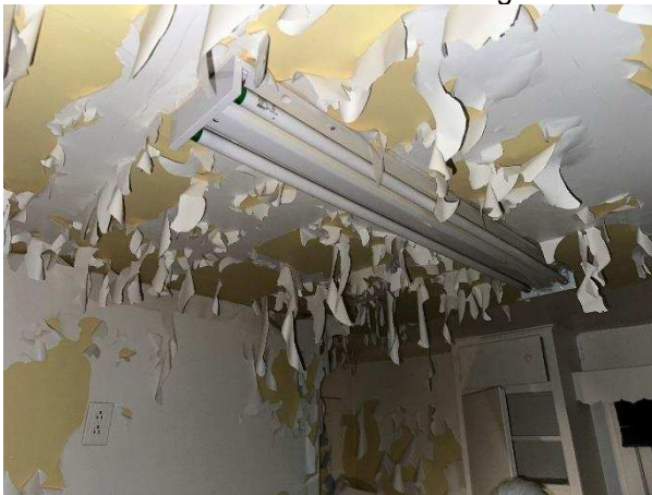
Photo 7: Interior finishes deterioration
