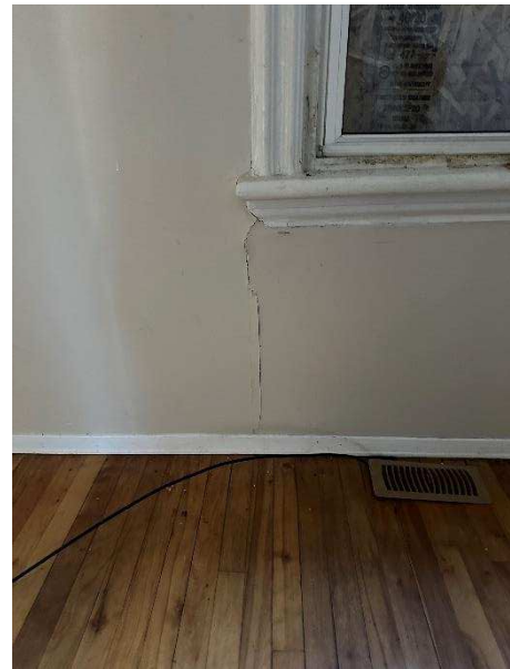
Photo 8: Interior cracking in finishes at window
