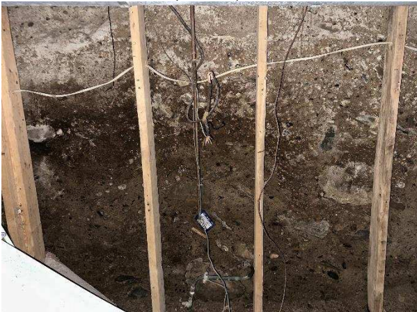
Photo 19: Foundation wall Water ingress and deterioration (interior)
