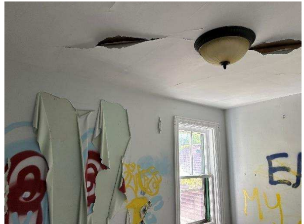
Photo 4: Interior paint peeling and ceiling damage
