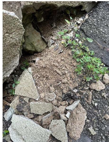
Photo 12: Concrete foundation deterioration at grade (exterior)
