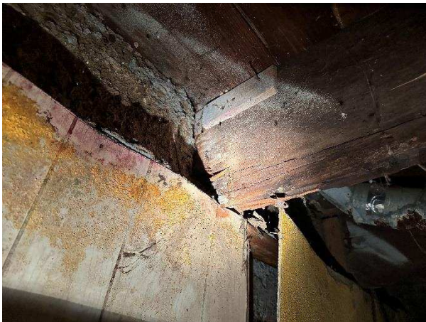
Photo 15: Unsupported wood floor beam
