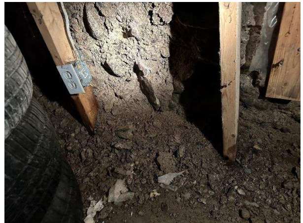
Photo 16: Concrete foundation deterioration (interior)
