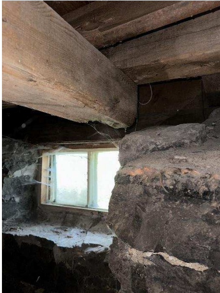
Photo 9: Primary ground floor beam shifted and unsupported
