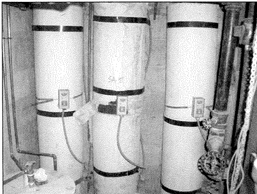
Photo 6 - Friable asbestos boiler insulation, basement 138 Bank Street.
