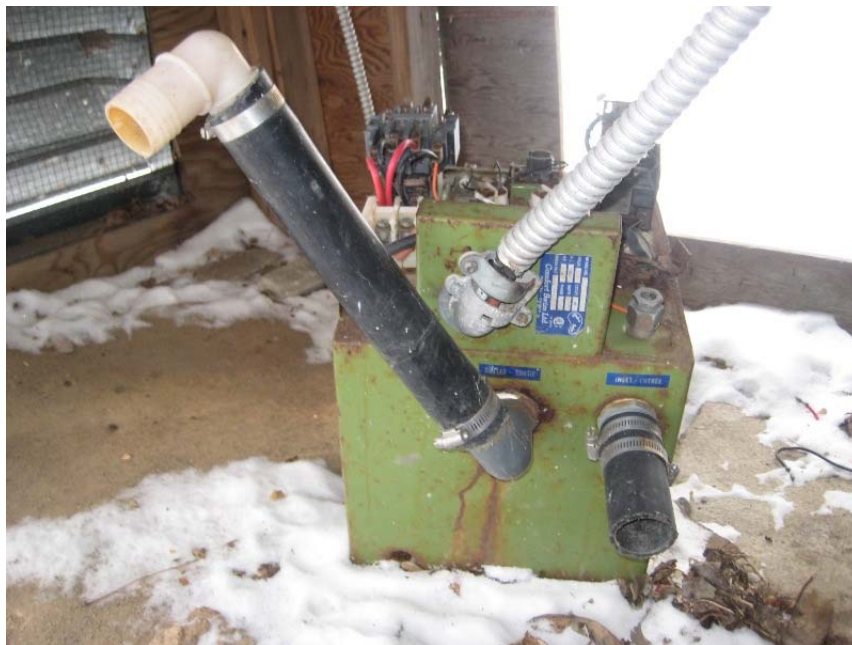
Photograph 8: View of a heating apparatus found underneath the exterior stairs, with visible electrical input and pipes for liquid input and output. This is thought to be associated with a former swimming pool on Site.
