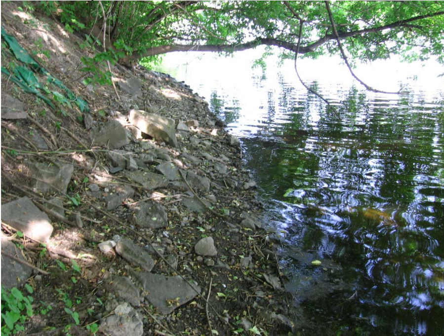
Photo 13. Shoreline showing broken concrete and unconsolidated material that has been moving downslope toward the river. While the Manitoba maples provide overhead shade, the shoreline itself lacked riparian vegetation – May 25, 2010.
